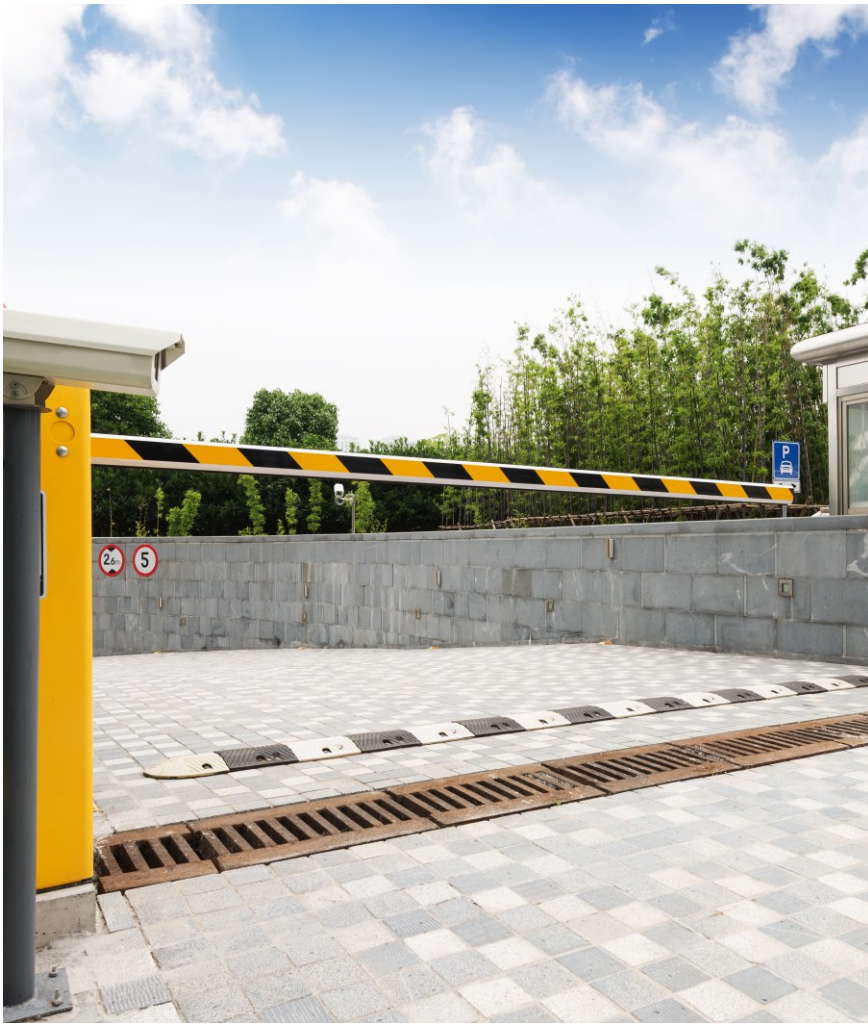
Automatic boom barrier Entry/ Exit
