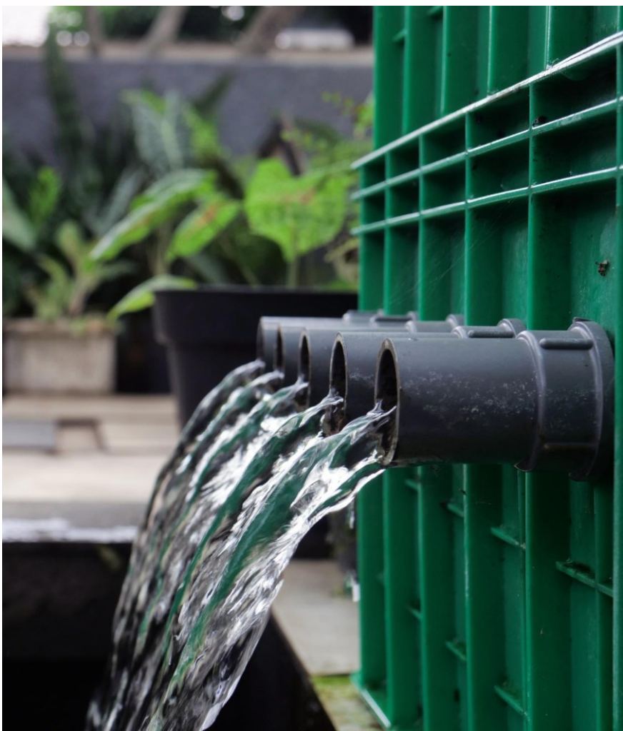
Rainwater Harvesting System
