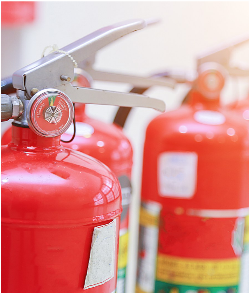
Fire fighting system
