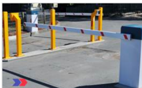
Automated Boom Barrier
